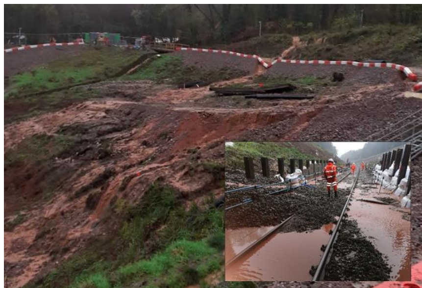
Plate 9. Honiton Tunnel Portal washout 21.11.2022
