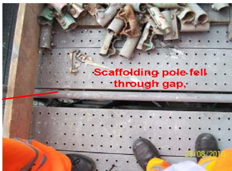
Plate 21: Clear gap in protection deck caused safety incident
