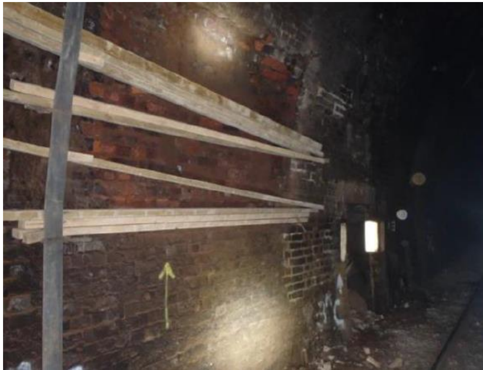
Plate 24: Temporary works in tunnel struck by train.
