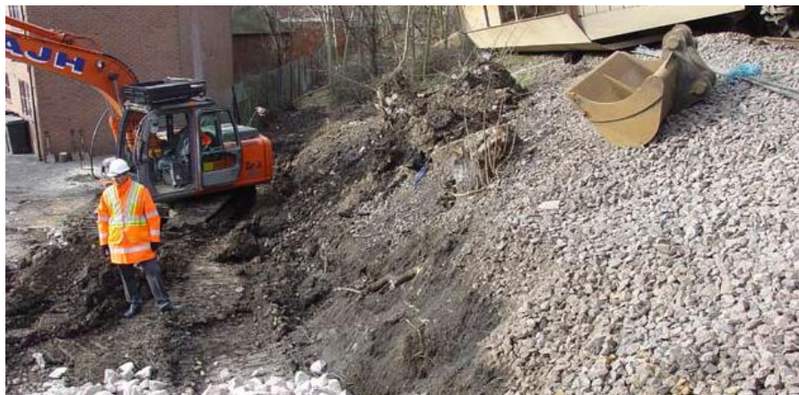
Plate 29: Temporary excavation to create works access road and site of derailed freight train at Cricklewood.
