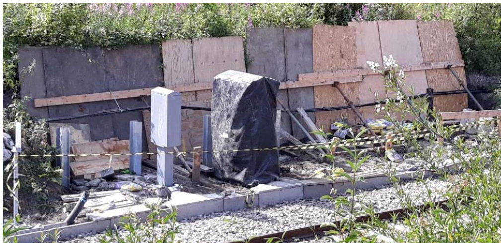
Plate 28: Breich, Scotland. Very poor Temporary Works with no design.
