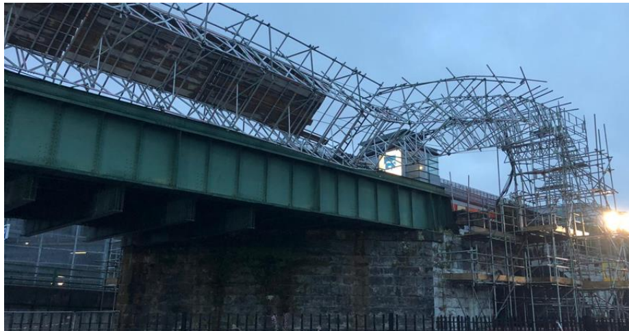
Plate 15: Warrington Scaffold bridge failure MAJ1,
