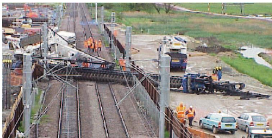
Plate 16: LTS line crane failure due to inadequate foundations.
