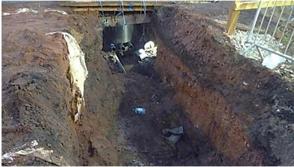
Plate 27: Stafford trench collapse due to no temporary shoring.
