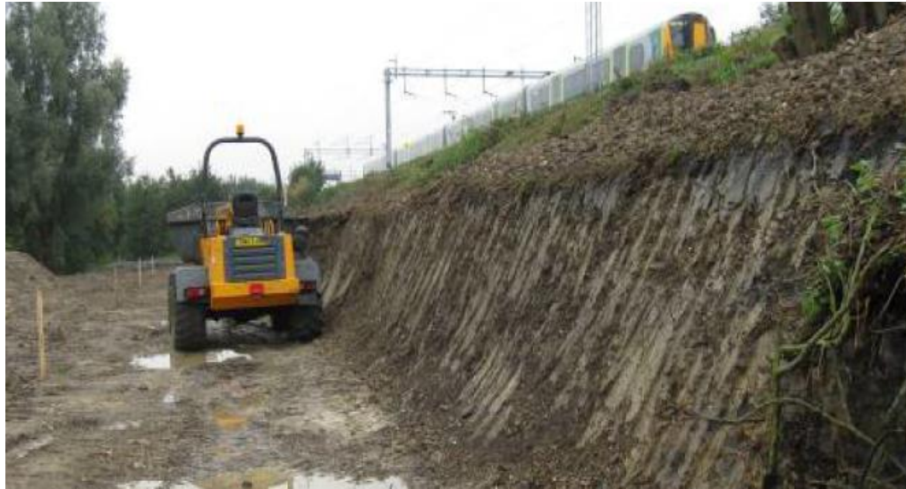
Plate 30: Bradwell Abbey toe cut contrary to (emerging) design, affecting track geometry (15 October 2013)
