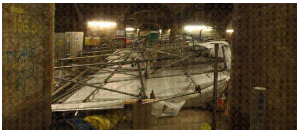
Plate 14: London Bridge Scaffold overturn 28.1.2015
