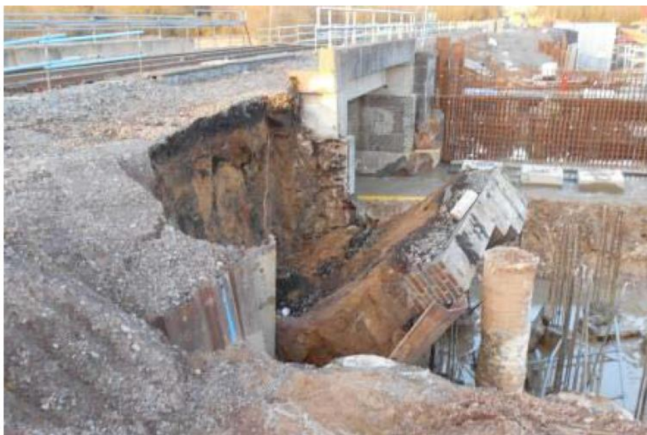
Plate 26: OXD39 Wingwall Failure due to undermining of existing structure during Temporary Works excavations.
