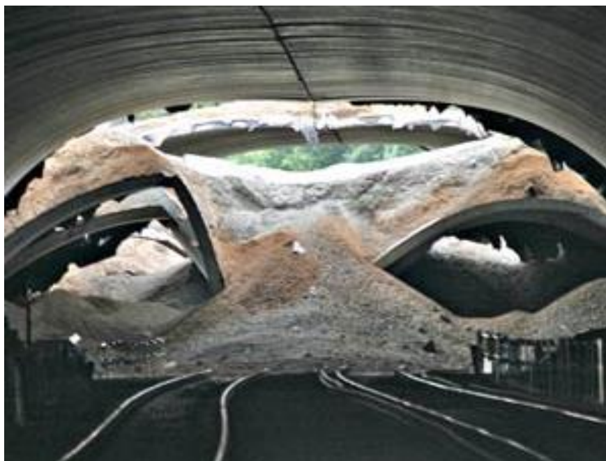
Plate 6: Collapse of Gerrards Cross Tunnel during construction.
