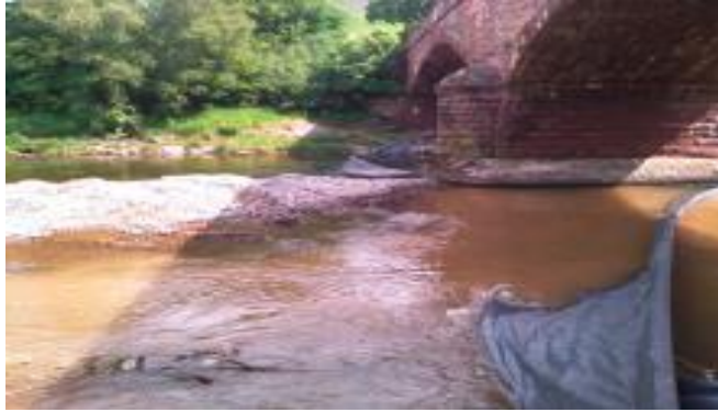
Works were halted but newly implemented mitigation measures at site and downstream were unable to contain sediment
