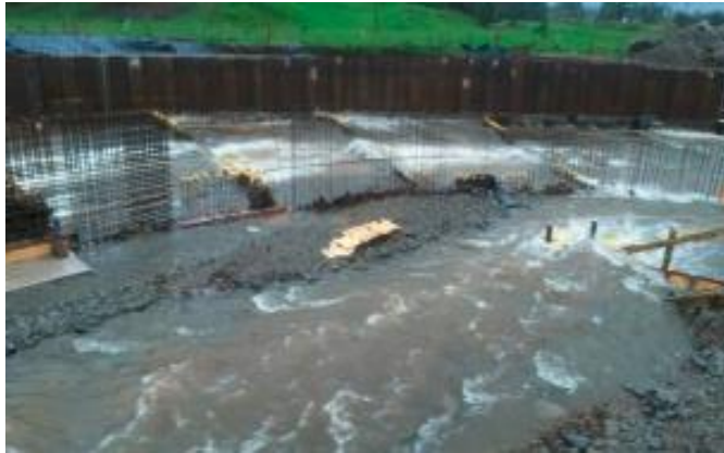
The temporary dam at diversionary channel was overtopped, which resulted in flooding of worksite in the permanent channel
