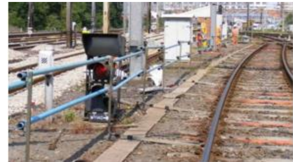
Temporary fence obstructing signal
