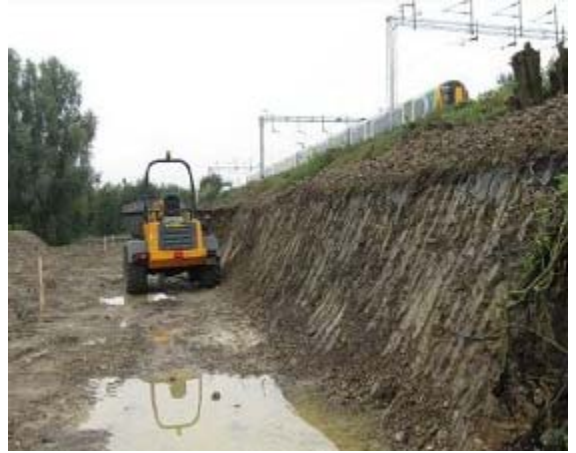
Toe of embankment removed without support
