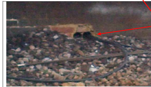
Trackside cables running into switch room through ducting
