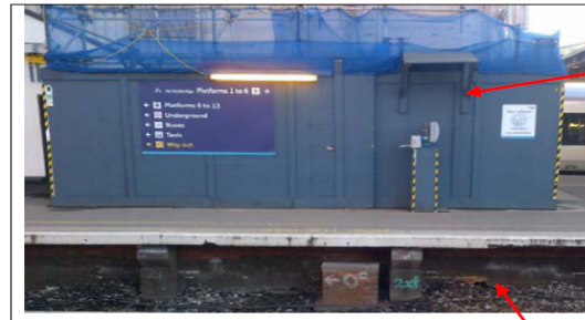
The switch room is located behind the hoarding
