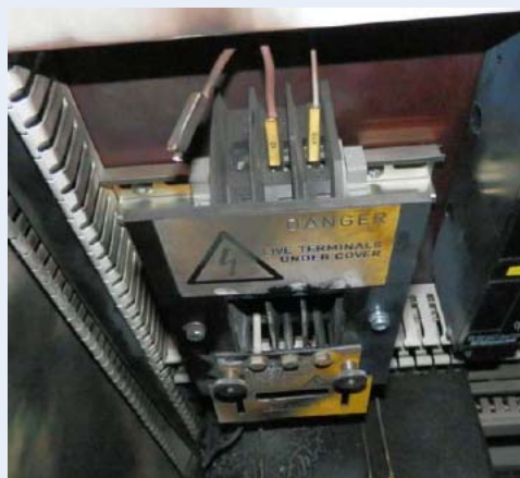
(ii) Flashover damage to equipment
