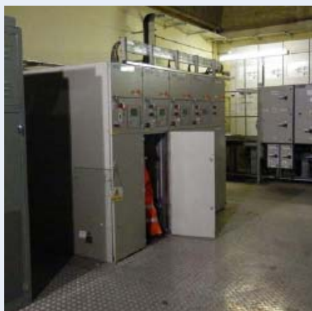
(i) Circuit Breaker housing
