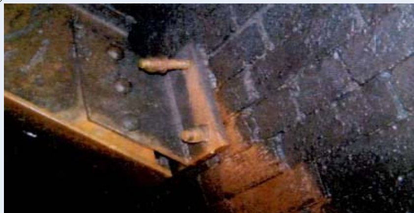
Photograph of failed stud
