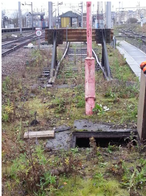
Above: Existing Brick Chamber UTX, light and buffer stop.
