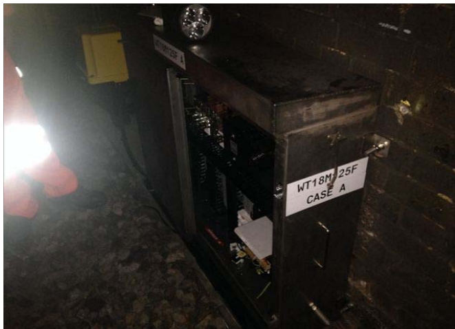
Location case with door missing
