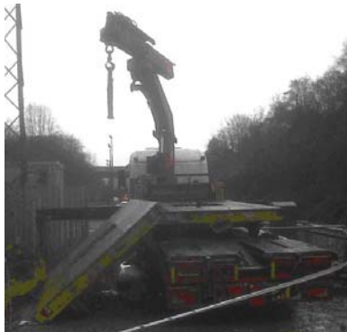
3-tonne trailer dropped from crane
