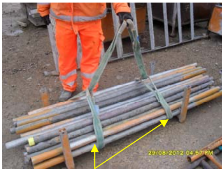
Load was secured with straps in between 2 unconnected scaffold storage frames
