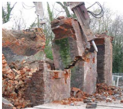
Collapsed arch at Beenham Lockside
