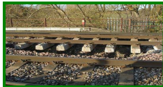
Figure 3: Visible damage under track
