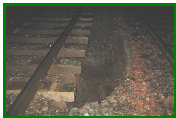
Figure 1: Hole in Ballast
