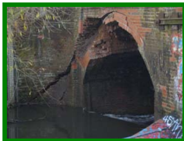
Figure 2: Damage to structure
