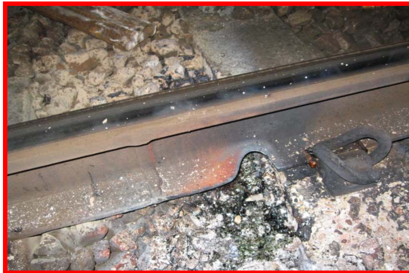
The burn marks to the running rail resulting from the flashover
