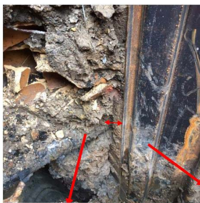
22KV cable found Friday 14th Oct
