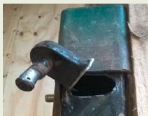
Photo of top hinge of gate that failed
