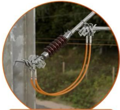
Circuit Main Earth
