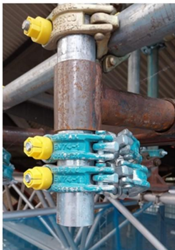
Revised detail with swivel coupler fittings permitting visual inspection of both fittings by erector. Note: Yellow Clickon caps to aid inspection.
