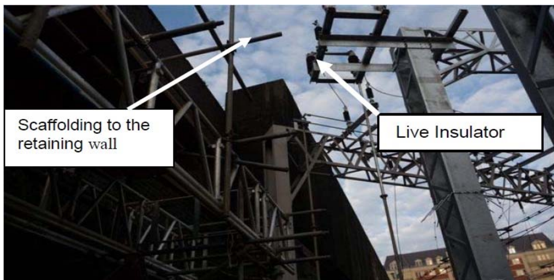
Plate 17: Scaffold constructed within 500mm of live overhead line equipment. Remedial works led to delay and disruption
