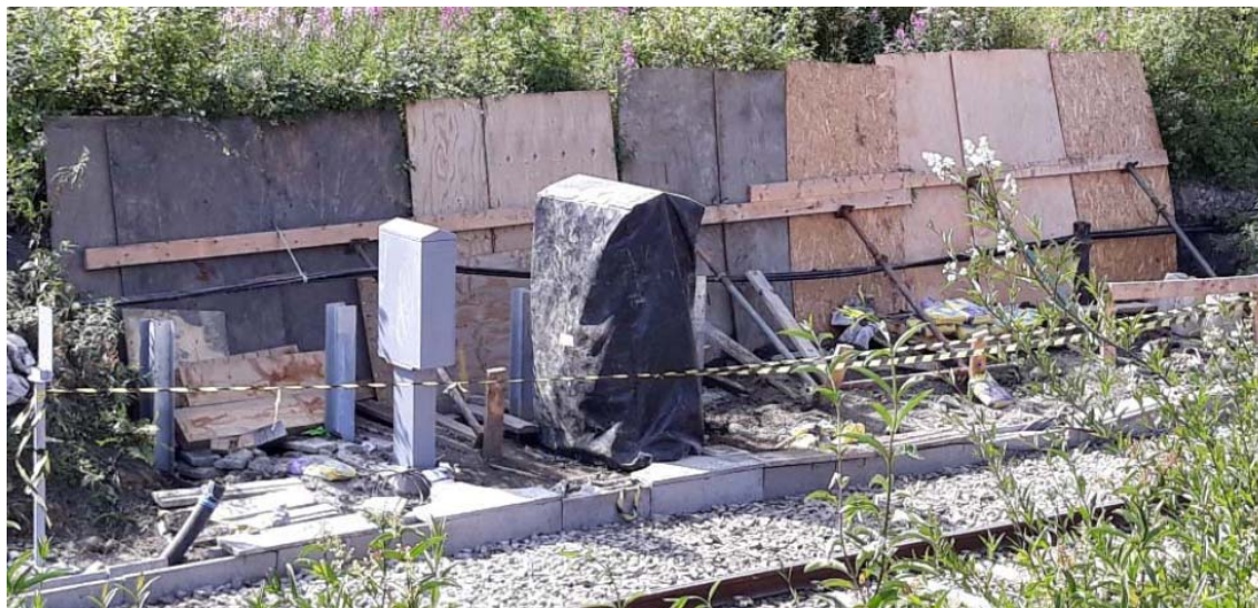
Plate 23: Breich, Scotland. Very poor Temporary Works with no design.
