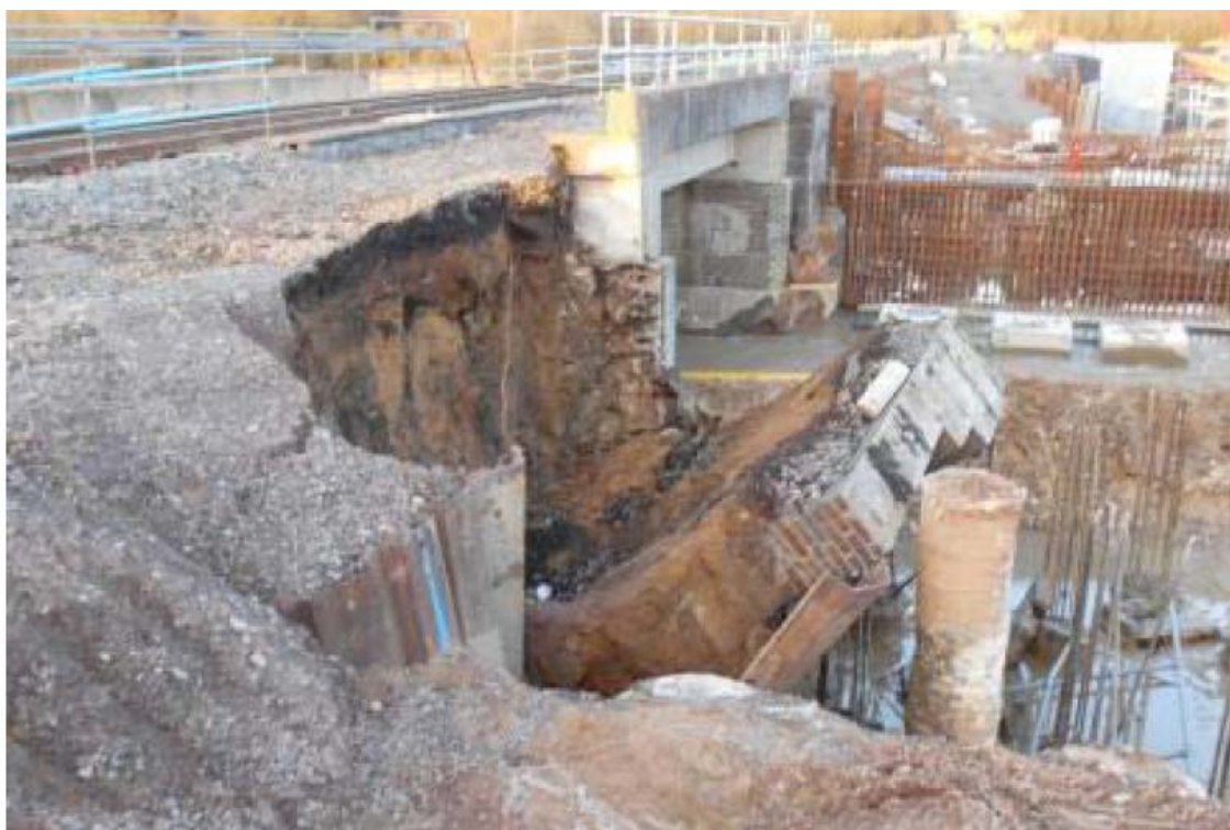
Plate 21: OXD39 Wingwall Failure due to undermining of existing structure during Temporary Works excavations.
