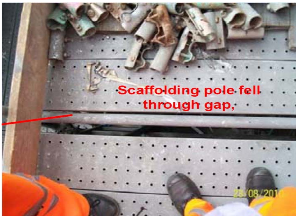
Plate 15: Clear gap in protection deck caused safety incident
