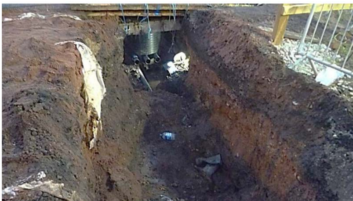
Plate 22: Stafford trench collapse due to no temporary shoring.
