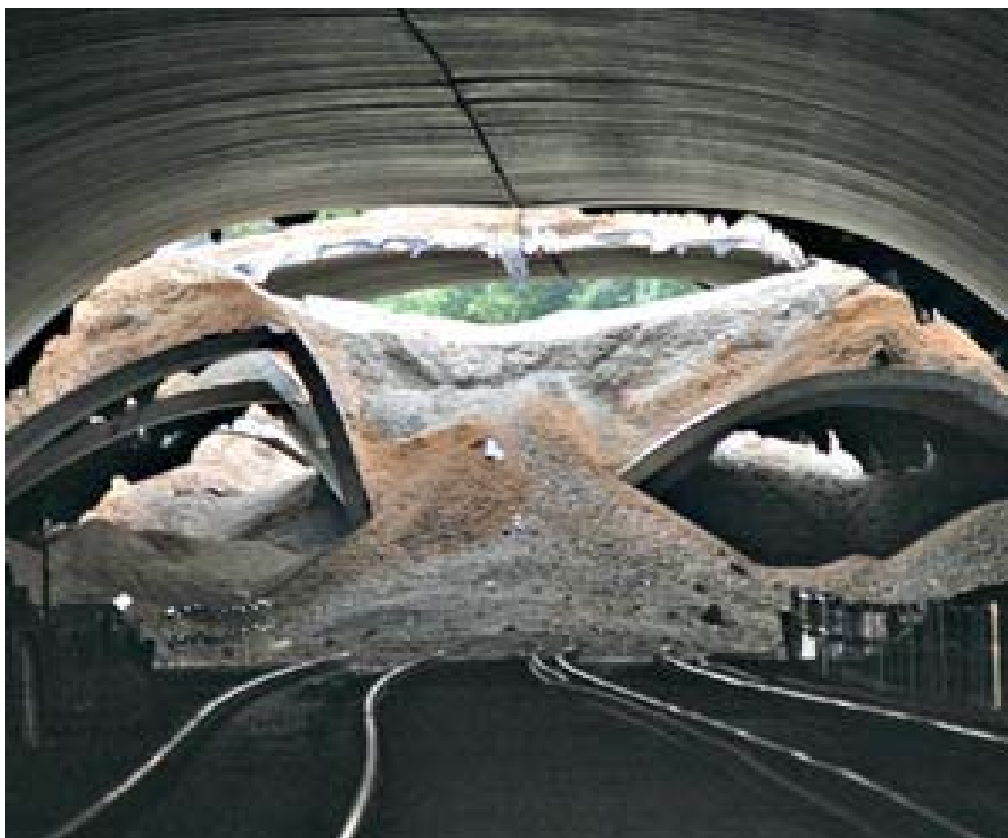
Plate 6: Collapse of Gerrards Cross Tunnel during construction.
