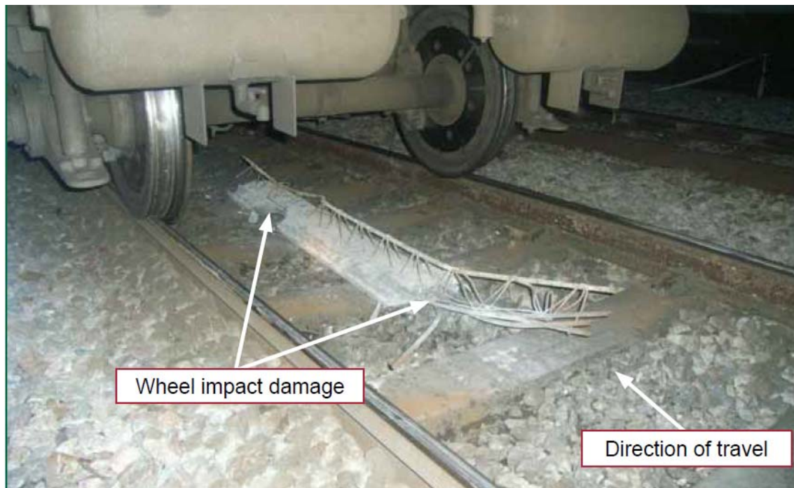
Plate 8: GE19 showing failed components having fallen from bridge over.
