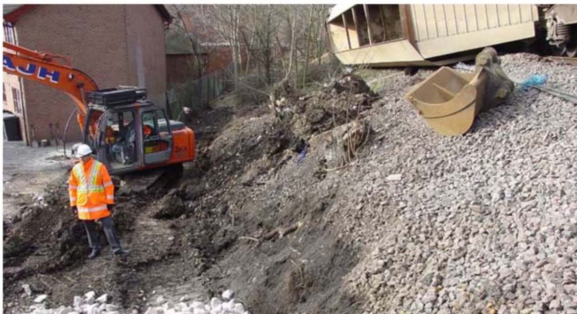
Plate 24: Temporary excavation to create works access road and site of derailed freight train at Cricklewood.
