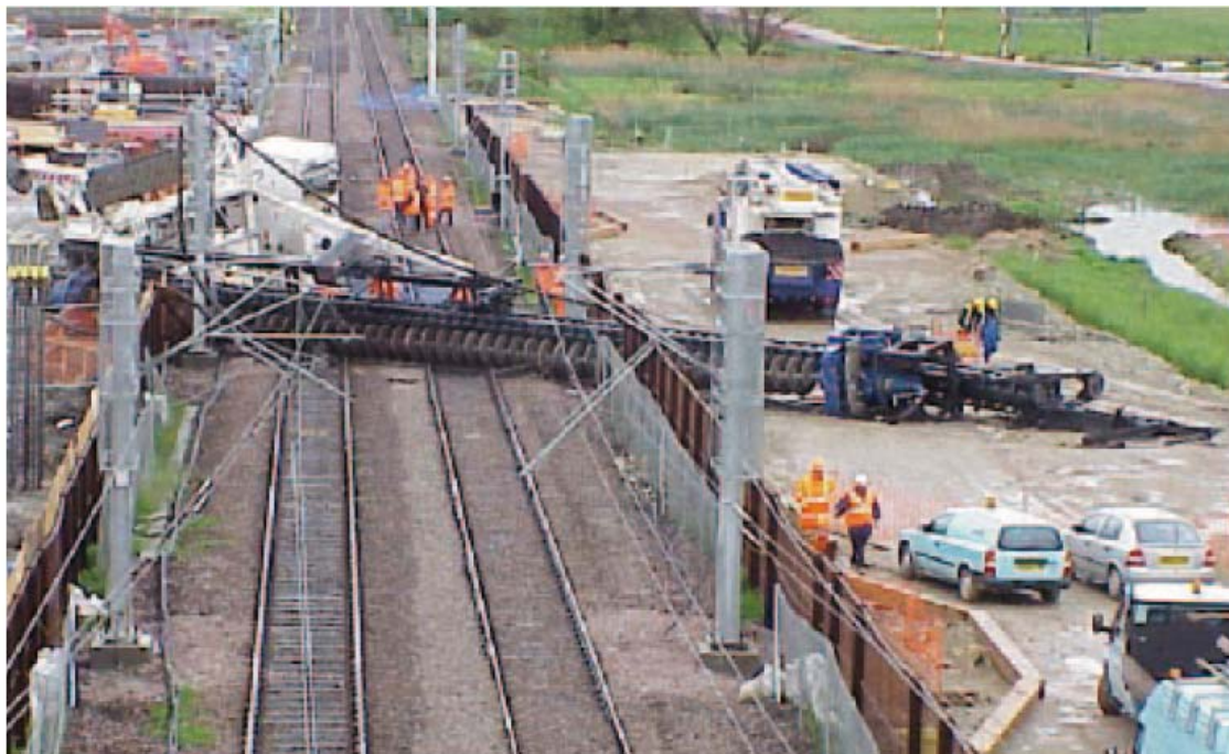
Plate 10: LTS line crane failure due to inadequate foundations.
