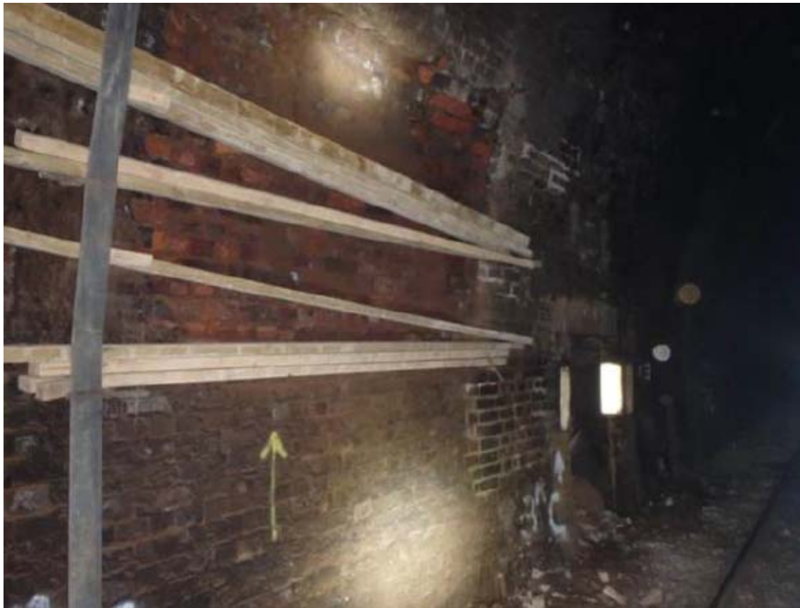
Plate 19: Temporary works in tunnel struck by train.
