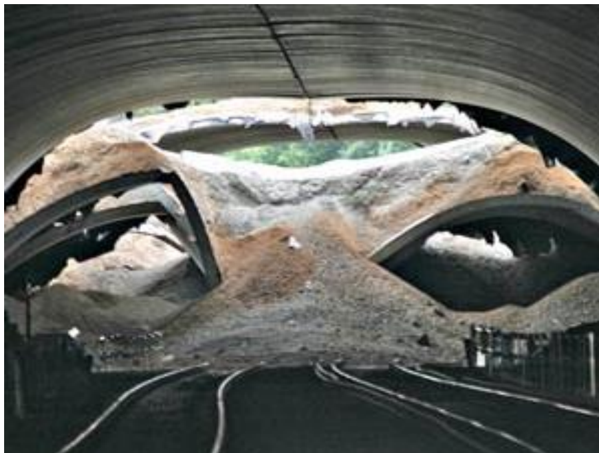
Plate 6: Collapse of Gerrards Cross Tunnel during construction.
