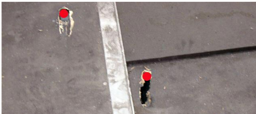
Plate18: Protection Deck Penetrated by Dropped Loads.
