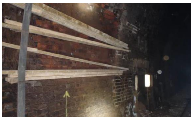
Plate 24: Temporary works in tunnel struck by train.
