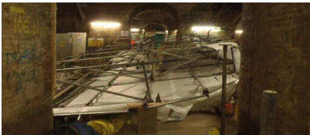
Plate 14: London Bridge Scaffold overturn 28.1.2015
