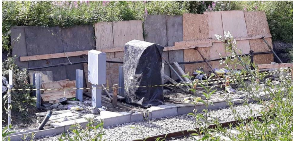
Plate 28: Breich, Scotland. Very poor temporary works with no design.
