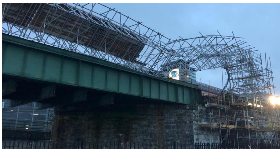
Plate 15: Warrington Scaffold bridge failure MAJ1,
