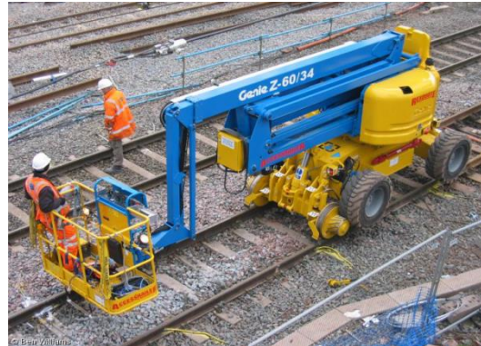
Mobile Elevated Work Platform (MEWP)
