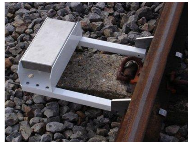
APC Magnet, installed in pairs before and after neutral sections.
