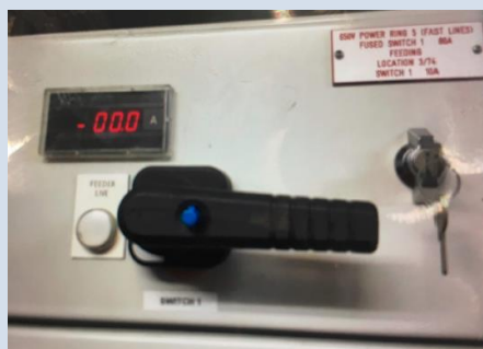
Photo of Switch :
