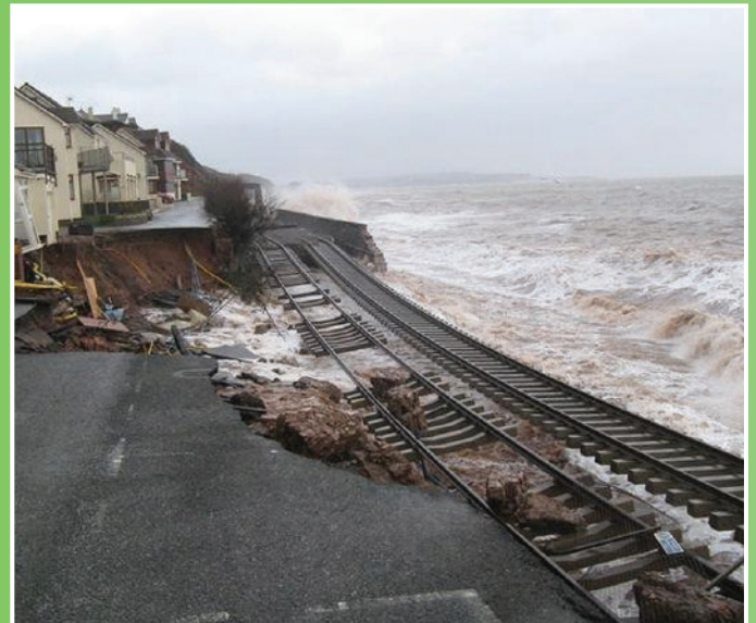
(Above) Dawlish, February 2014 showing how important our weather resilience and climate change adaptation plans are at preventing incidents like this
