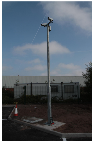
CCTV installed on a hinged pole within car park
