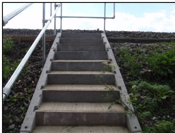
Stanton & Bonna stairwell built on an embankment (Type 1 stone or concrete infill)
