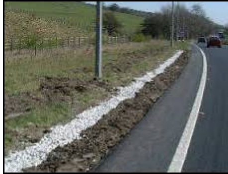
Filter drain installed along a typical roadway.
