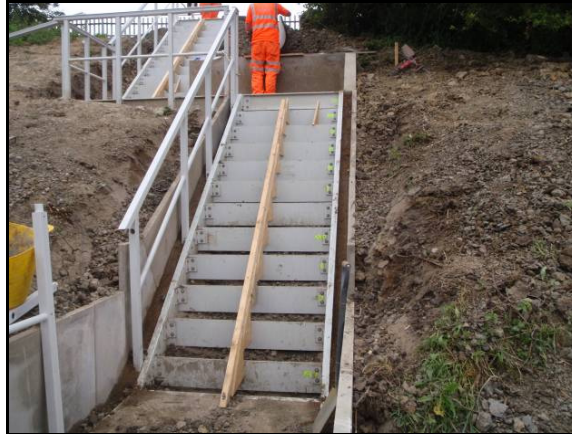
GRP / FRP steps on a cutting slope
