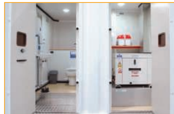
Easily accessible generator
