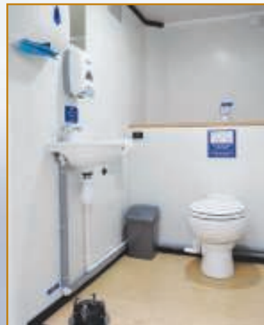
Toilet facility with hot and cold running water
