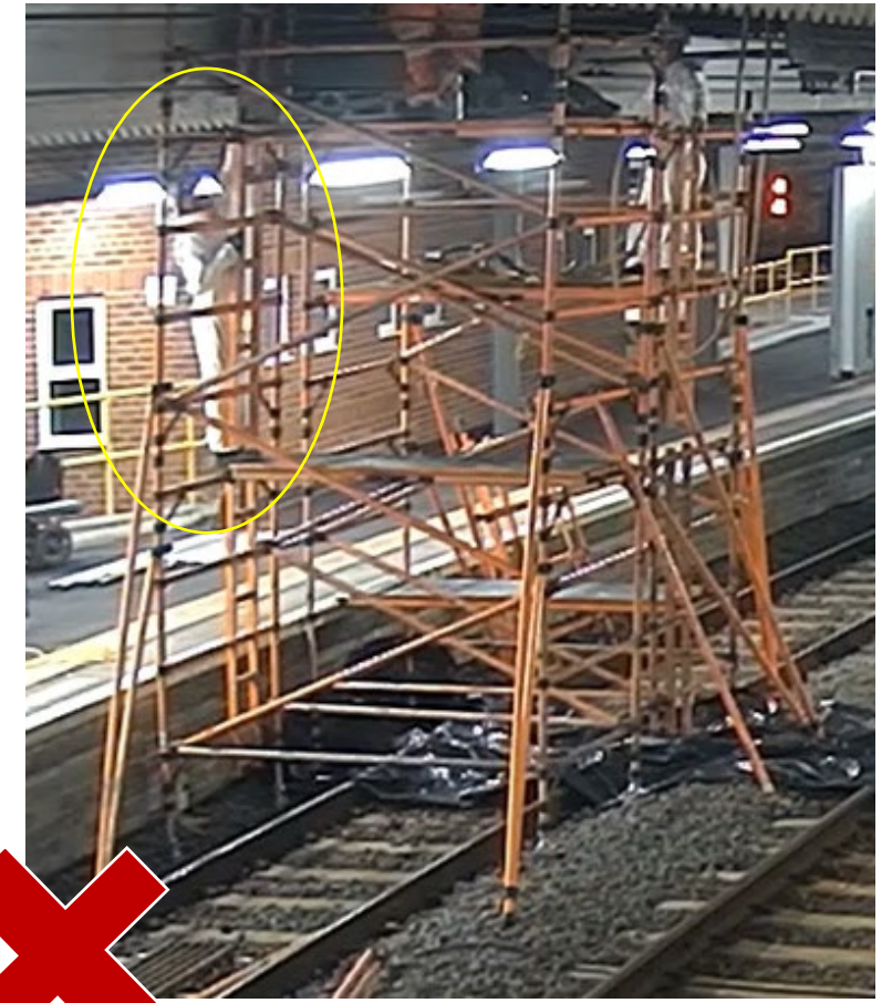
Climbing up outside of mobile tower.
