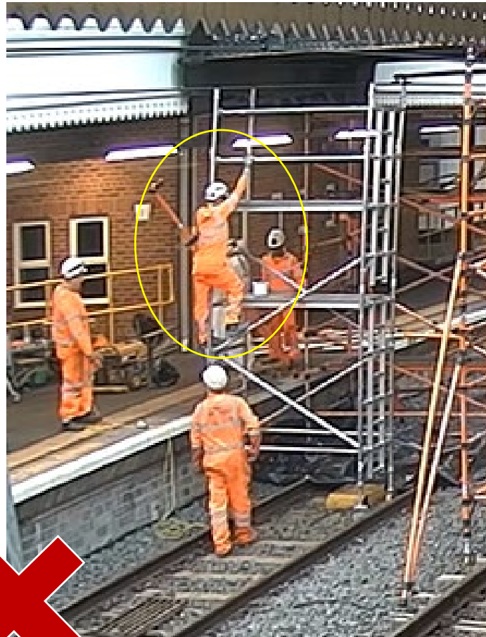
Climbing up outside of mobile tower.
