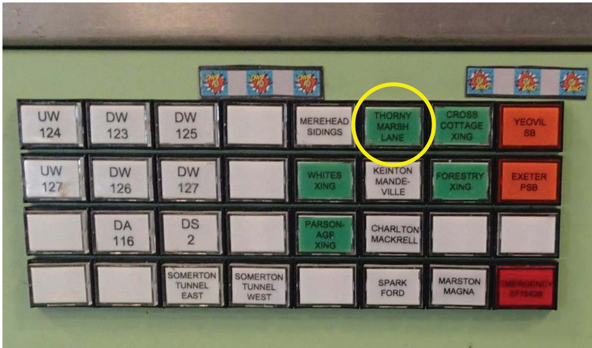
Telephone concentrator on signaller's control panel. Button for Thorney Marsh Lane crossing circled
