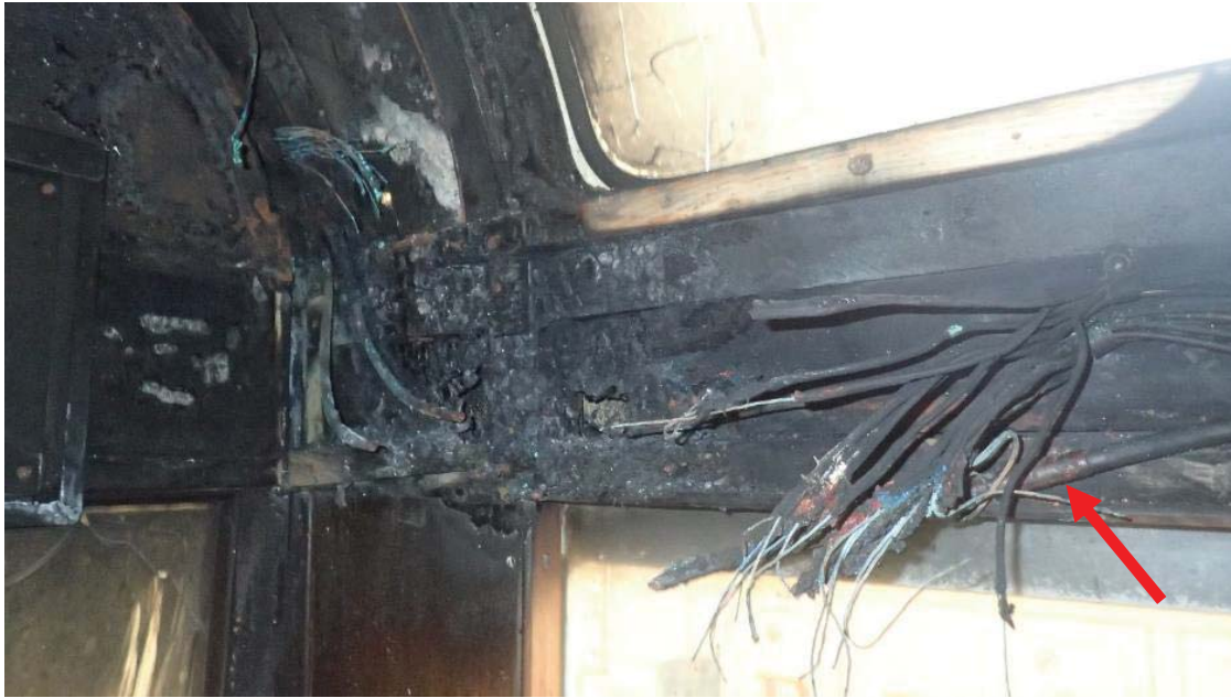
Fire damaged cabling within 272; the previous cable repair is indicated by the arrow
