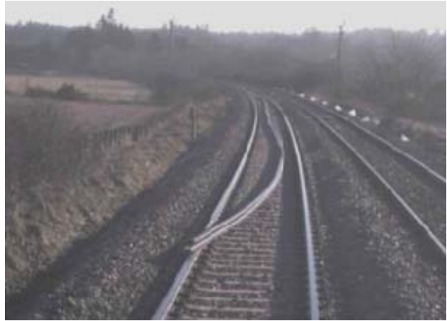
Footage from train mounted FFCCTV
