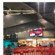
Exclusion zone set up in concourse after the panel fell
