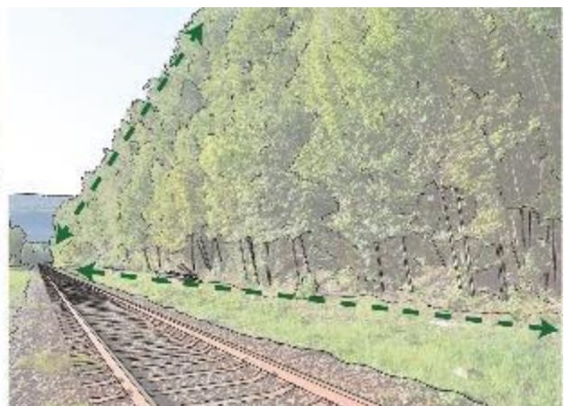
Figure 23b – After vegetation management. There is evidence of tree felling and the cess strip is clear of any vegetation
