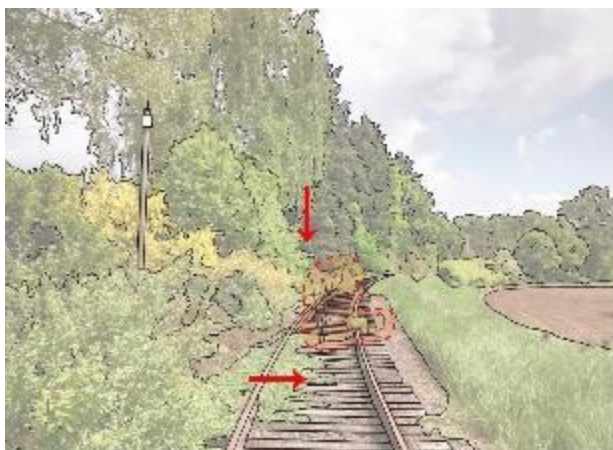
Figure 23a – Before vegetation management. Vegetation is creeping onto the track and over-hanging branches are a safety risk
